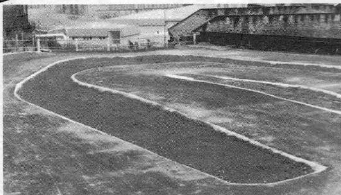
Below: the tarmac is down and run-off areas designated, these will be grassed over in due course. That wide sweeper looks fun!
